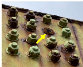
Figure 202. Broken bolt on south truss of upper gusset near midspan of centre span (photo from HHB)
