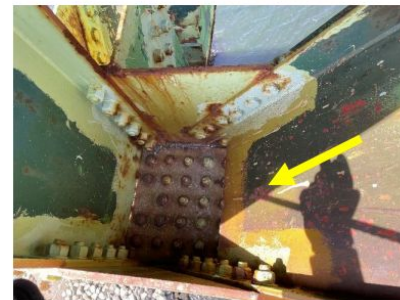
Figure 24. Example diagonal deterioration near the lower truss nodes
