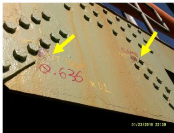
Figure 56. Maximum measured pitting depth of approximately 3.2 mm – S-WS-U1
