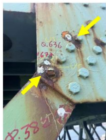
Figure 55. Maximum measured pitting depth of approximately 3.2 mm – S-ES-U51
