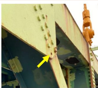
Figure 203. Missing bolt on south two bays east of prior photo in Centre Span (photo from HHB)
