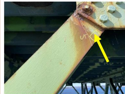
Figure 23. Example of a gusset with rust staining due to upper gusset above
